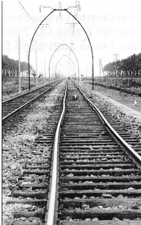
Figure 4 - Railway track after the first high speed test by SNCF[30].
