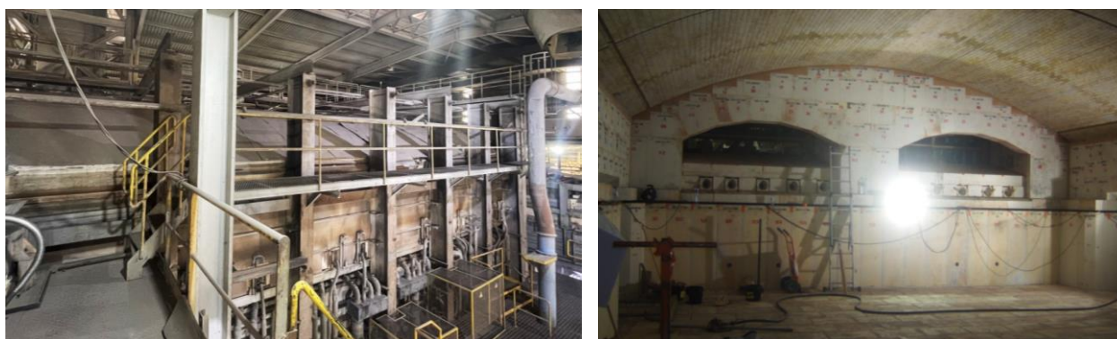
Figure 10 - Furnace facility outside and inside views.
