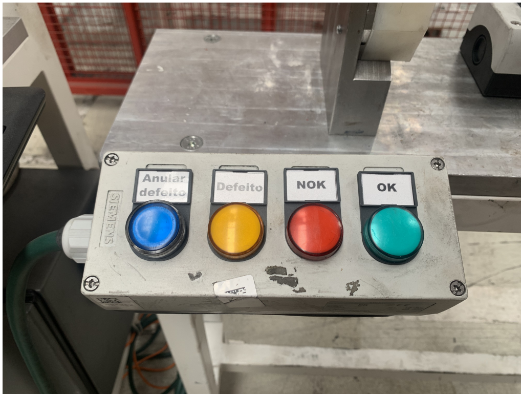
Figure 3.39: Control box, with light indicators and blue button.
