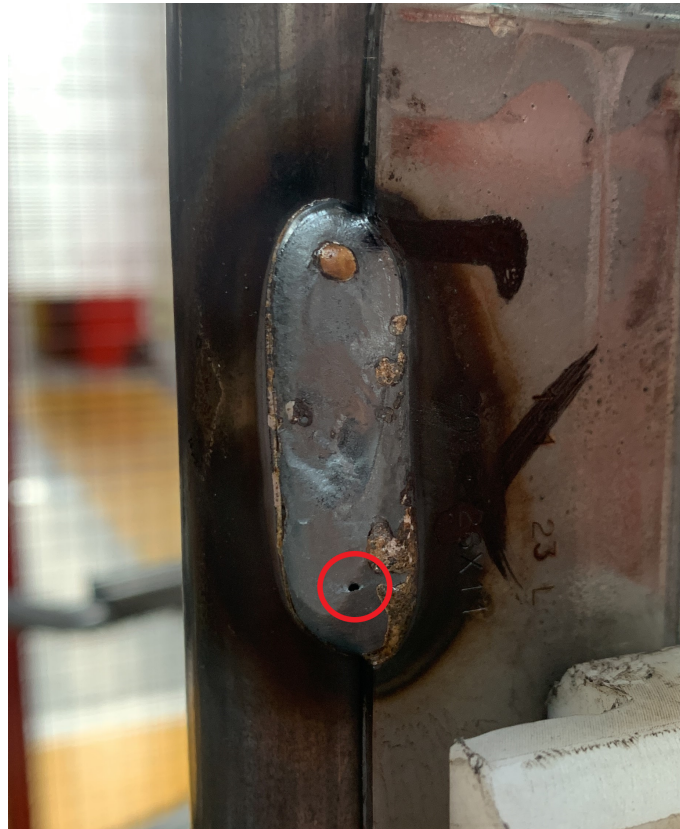
Figure 4.2: Porous weld 8 from part 10.
