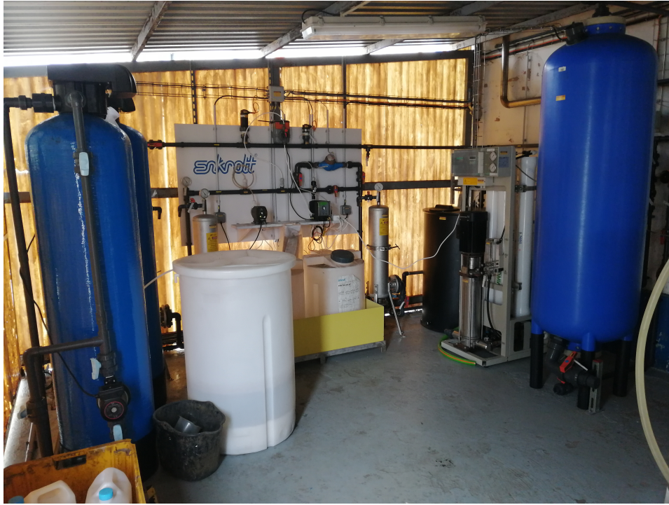
Figure 3.9: Reverse osmosis process in the plant
