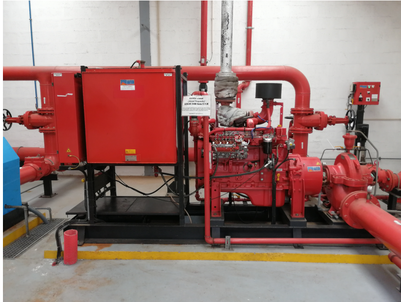
Figure 3.6: GOULDS 3408 8x6x12 F-M diesel pump
