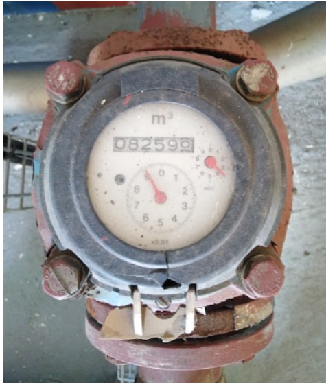
Figure 6.3: Reverse Osmosis PT meter
