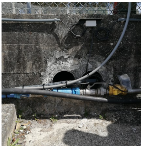
Figure 6.2: Electrovalve placed next to the factory's entrance
