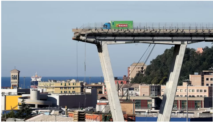
Figure 1.2: Colapse of the Morandi bridge in 2018 [2]
