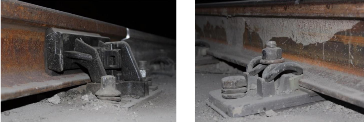
Figure 3-3 - Examples of direct fastenings (left) and indirect fastenings (right). Taken from Sadeghi et al. (2020)
