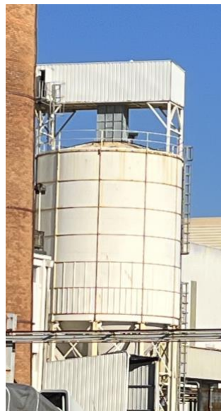
Figure 3.2: Silo for sand storage
