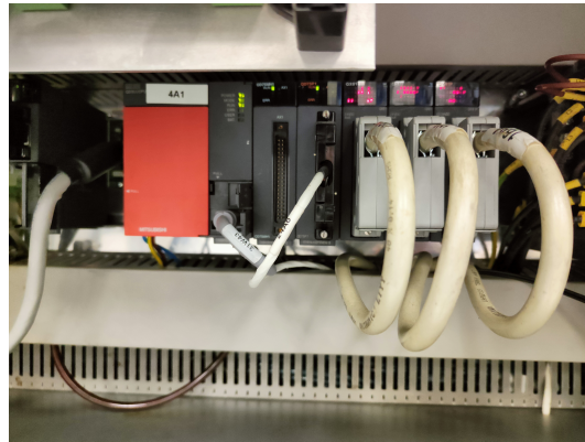
Figure 2.10: PLC on the ICT module
