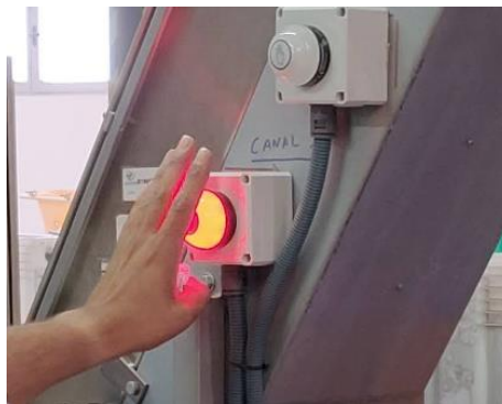
Figure 51 - Operator pressing the illuminated pushbutton installed
