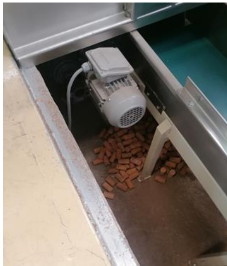
Figure 58 - Conveyor ditch full of stoppers
