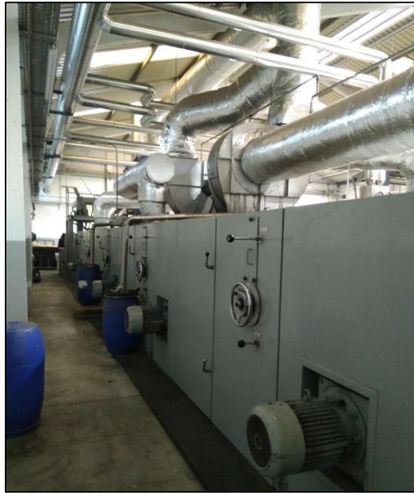
Figure 10. Heat setting machine used at ACATEL.
