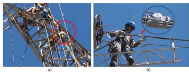
Figure 7. Accelerometers installed: a) piezoelectric (tower) and b) MEMs (conductor).
