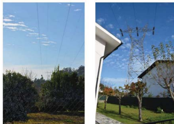
Figure 1. LRA.VM1 Line: a) span e b) instrumented tower.
