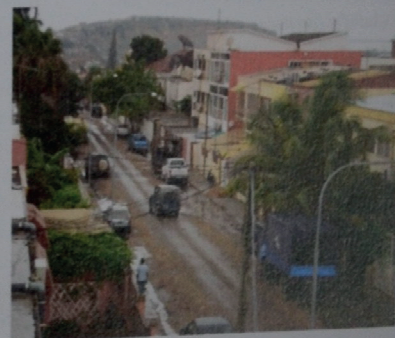
A street in Luanda in the rainy season, about two years ago, where one can see the poor state of the paving and the destruction of the footway.
