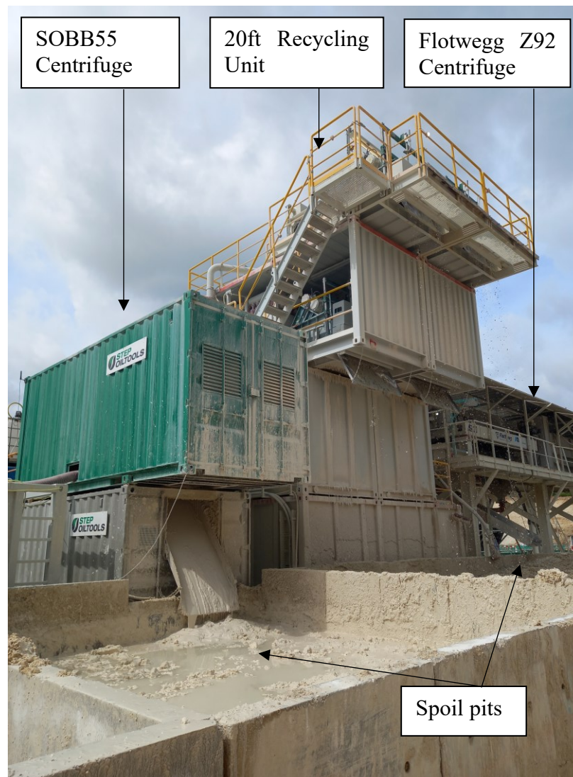
Figure 34: 20ft Recycling Unit and Centrifuges.
