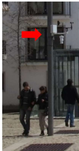
Figure 16. Example of an installed sensor (adapted from [17]).
