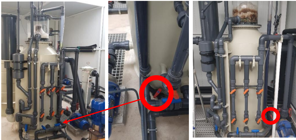
Figure 4 - Skimmers, and respective sewer valves;
