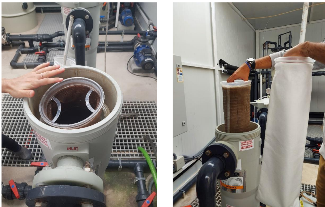
Figure 3 - Mechanical filter used and cleaned sleeves.
