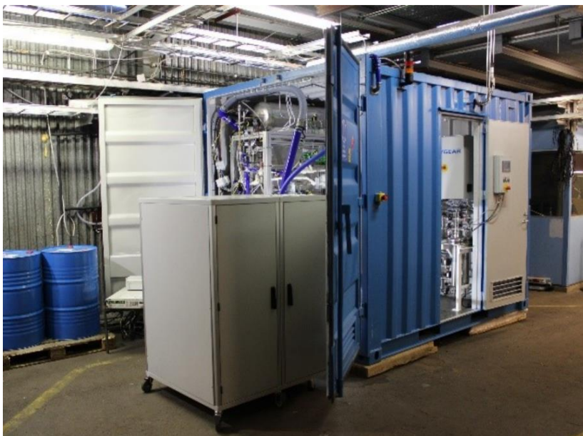
Figure B.5 – Picture of the reformed ethanol system container - outside
