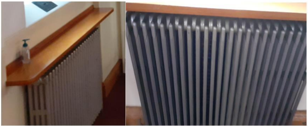
Figure 22 - Cast iron radiator
