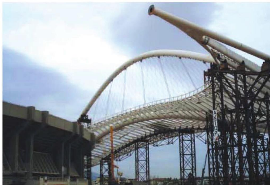
Tensoteci cable systems, Olympic Stadium, Athens
