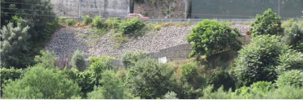
Annex 3 – Photograph of the risk analysis’ case study (i.e., a retention wall) taken from the opposite bank of the river.
