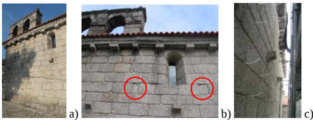
Figure 11. View of the Gondar church wall that exhibited out-of-plane deformations (a), view of two two-leaf stone connectors (b), injection of consolidation grouts (c).
