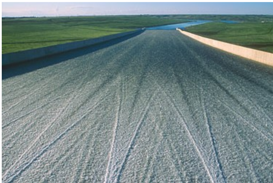
Fig. 13 – Cross-waves over the spillway of Gardiner dam, Saskatchewan, Canada, 1967 (copyright © Neil A Rawlyk).
