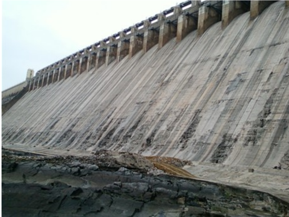
Fig. 15 - Cavitation damage in the Nagarjuna Sagar Dam, India, 1967 (from Giridhar et al. , 2014).
