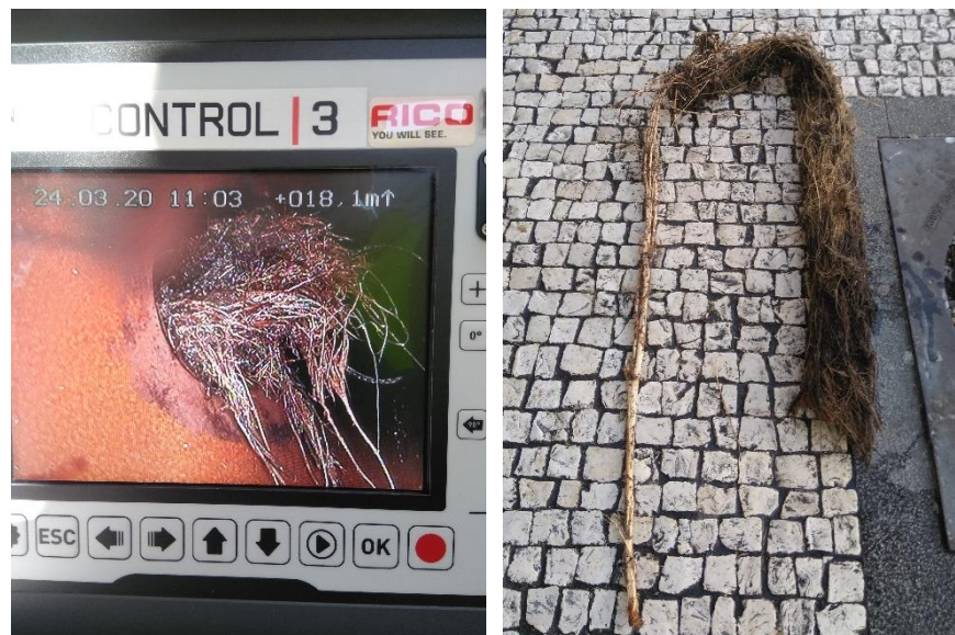
Figure 5: Tree roots observed inside a drainage pipe, through CCTV inspection (left) and the roots after removal (right) (Águas do Porto E.M. 2020)
