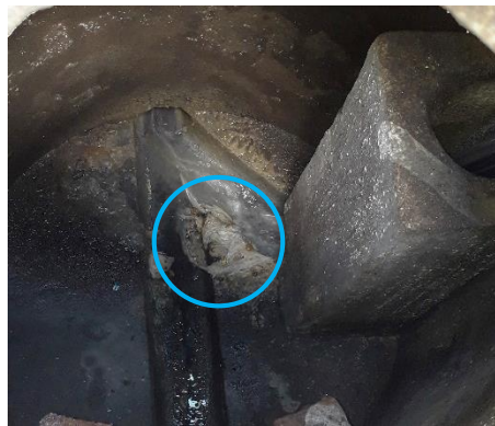
Figure 3: Debris build-up in the visitation chamber of a wastewater drainage network (Águas do Porto E.M. 2020)
