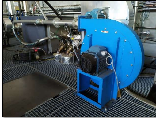
Figure 4.15 - Fan responsible for injecting air into the boiler.
