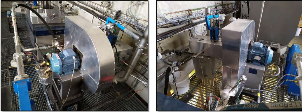
Figure 4.13 - Syngas extraction fan. The blue engine responsible for its working can be seen next to it, as well as the blue manual valve which initiates the extraction.
