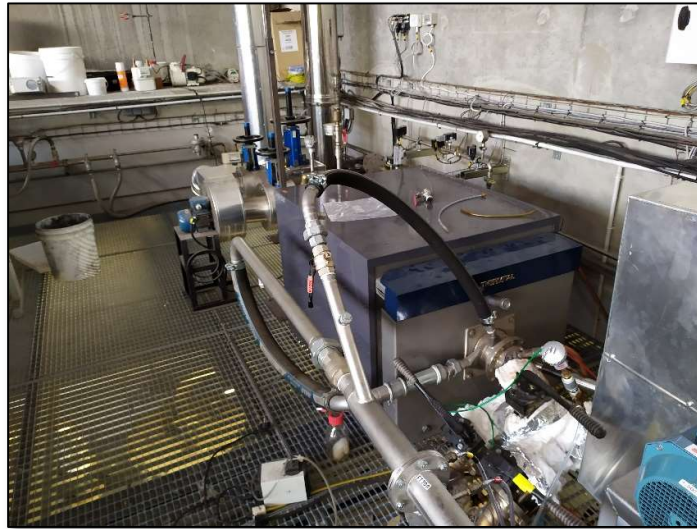
Figure 4.14 - Boiler where the syngas is burned to acquire energy. All the participants in the combustion are injected through the burner, seen here at the boiler entrance.
