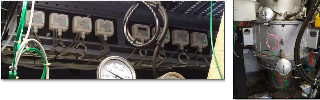
Figure 4.28 - Large amount of sensor data converters next to the gasifier (left). They collect measurements from the considerable quantity of sensors mounted on this part of the plant (right).
