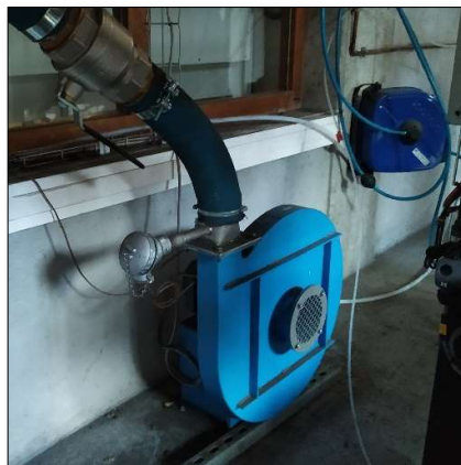
Figure 4.12 - Air injection fan - injects air into the heat exchanger to cool the syngas.
