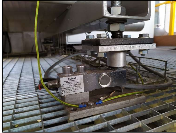
Figure 4.24 - One of the four weight sensors installed in the feed-hopper's legs.
