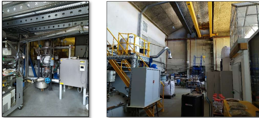
Figure 4.2 - Ground-level at PROVADEMSE’s gasification plant. The gasifier can be seen on the left picture.
