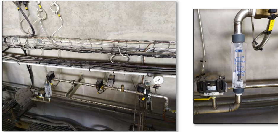
Figure 4.30 - Propane injection line (left). The flowrate is measured directly in the flowmeter (right).
