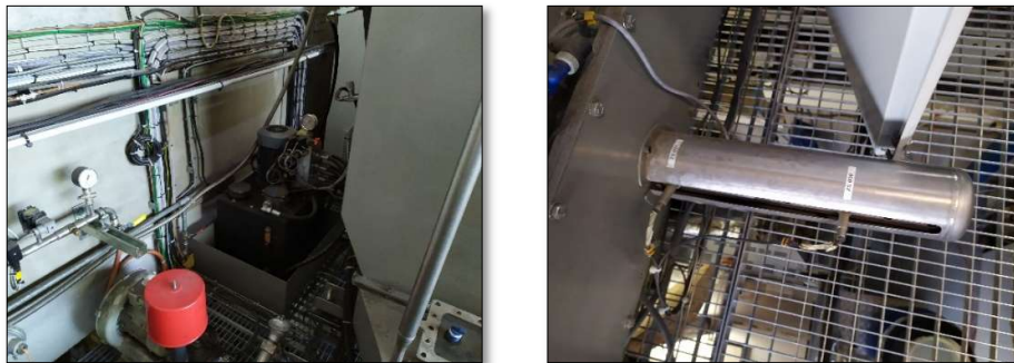
Figure 4.25 - Engine (left) that starts the hydraulically-acted (right) scraper which feeds the gasifier.
