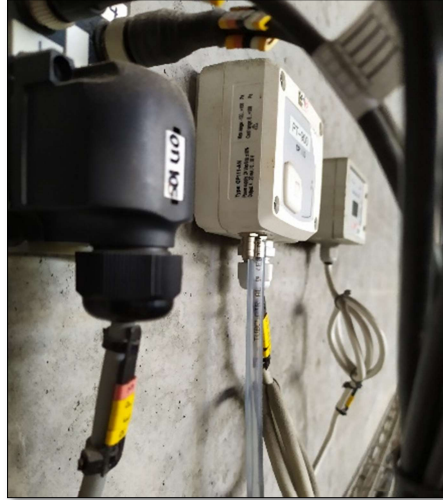
Figure 4.22 - Pressure sensor converter (centre).
