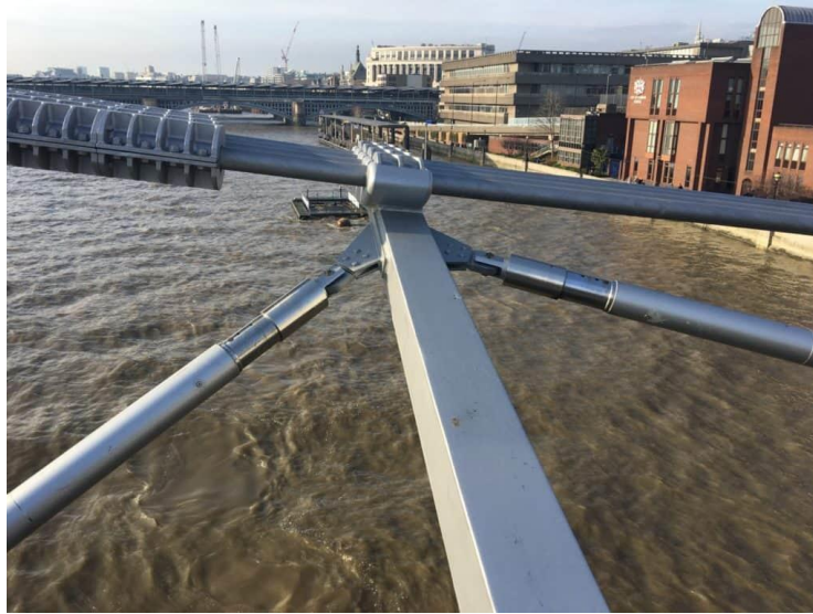
Figure 3 - Application of fluid viscous dampers on structures: Millennium London Footbridge [13].
