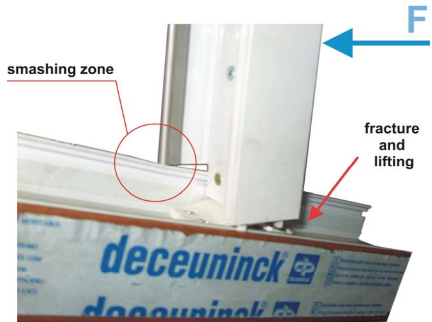
Figure 131. After fracture T junction in detail.
