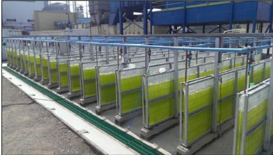
Figure 4 | Pilot facility of flat panel photobioreactors installed inside a thermoelectric power station located at Tocopilla (Chile) (Ación, 2017).
