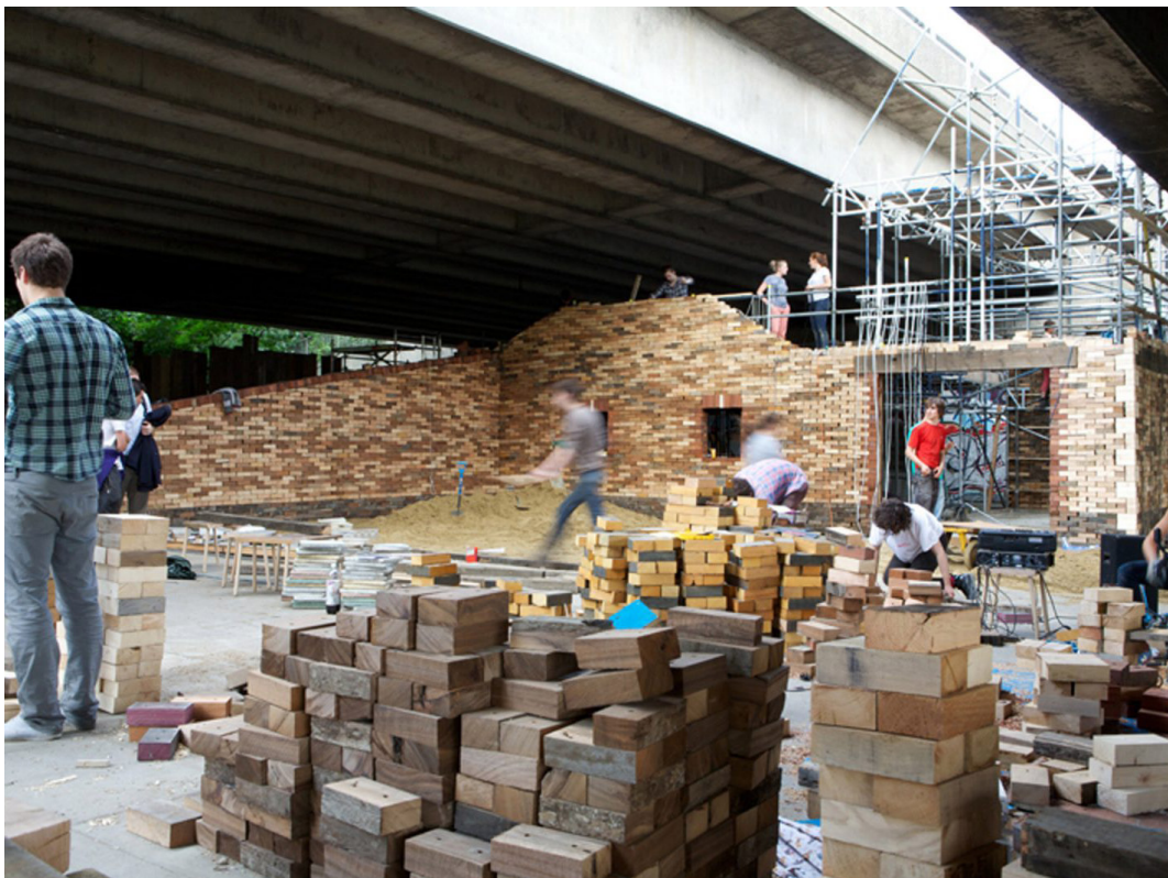
figura 58 Canteiro de obras de Folly for a flyover, fonte: https://assemblestudio.co.uk/projects/folly-for-a-flyover consultado no dia 27/08/2018
