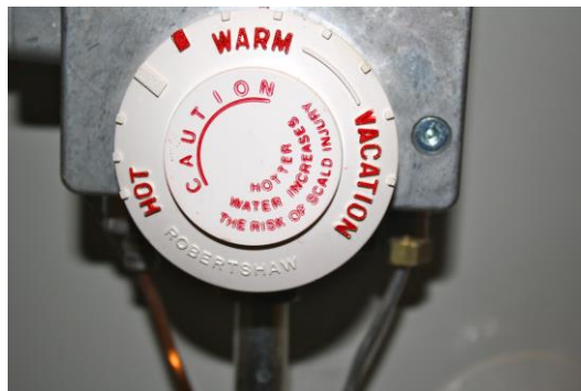
Figure 4 - Hot water heater regulator
