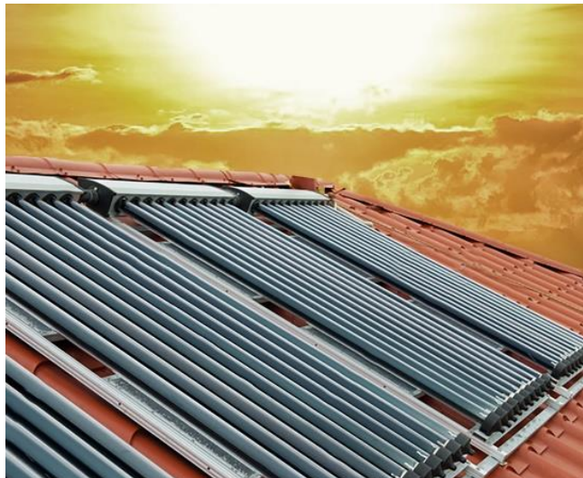
Figure 15 - Evacuated-tube solar collector mounted into a sloping roof. Extracted from [38].
