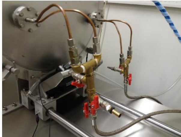
Figure 31- Copper tubing arrangement
