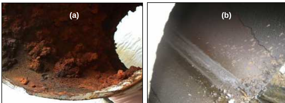
Figure 1.4 - Pipe sections from a drinking water distribution system made of (a) - ductile iron with high amounts of corrosion products and biofilm in Chaves (2004) and (b) - cement cast iron with high accumulation of biofilm and inorganic particles.
