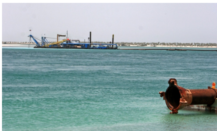
Figure 12 | Floating pipelines near the shoreline in Abu Dhabi
