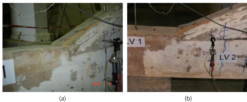
Figure 22. Evolution of wood local embedment in left rafter–tie beam joint: (a) fifth load cycle (60 kN); (b) seventh load cycle (80 kN)
