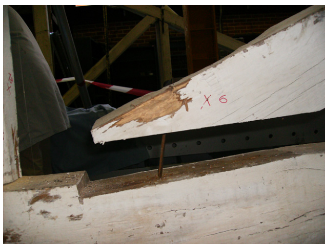
Figure 24. Opening of right strut-tie beam joint
