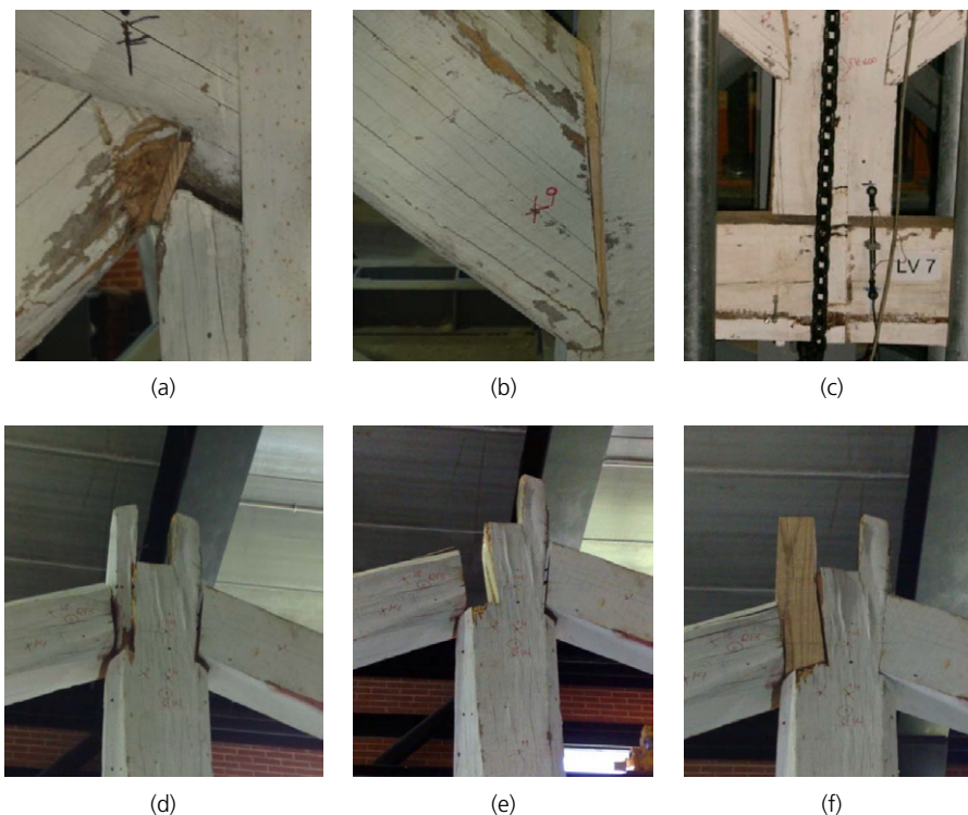
Figure 3. Reparation of some joints: (a) filling the gap with wood in a strut-rafter joint; (b) restoring the contact between connected surfaces in a strut-king post joint; (c) ensuring the separation
