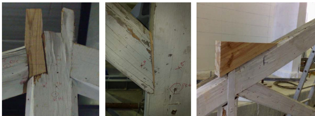
Figure 10. Carpentry works carried out to ensure a correct execution of the load-carrying test
