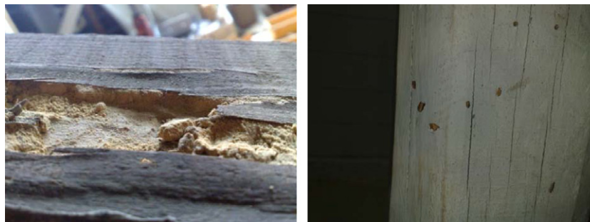
Figure 4. Superficial biological deterioration of timber caused by insects
