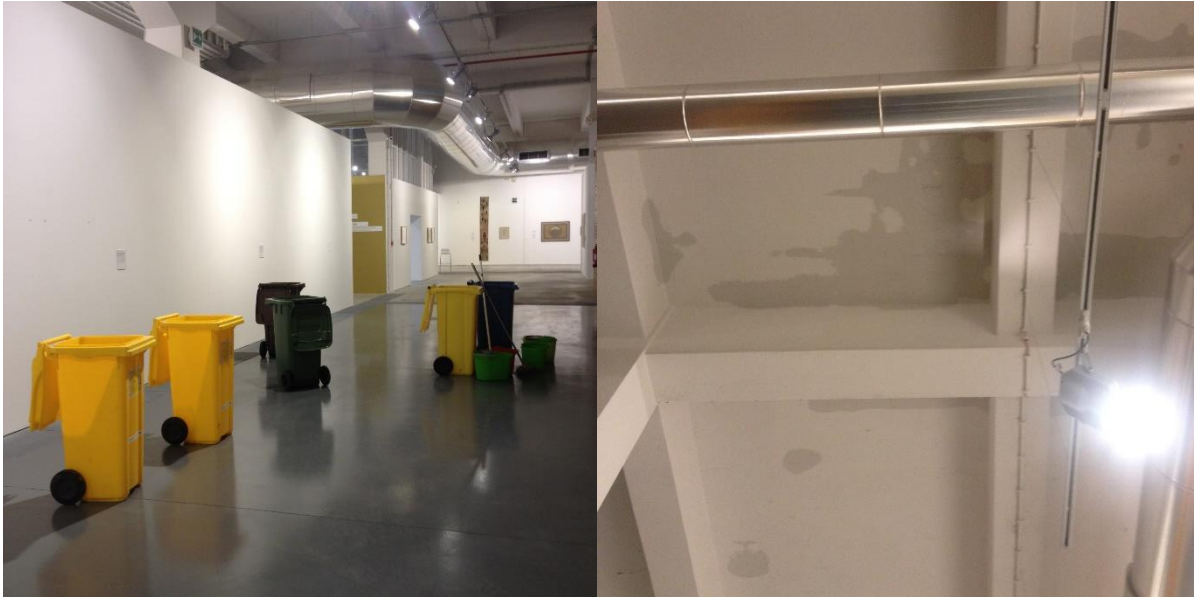
Fig. 41. The closed area of the exhibition damaged with flood and the view of the leak at the ceiling of Núcleo de Arte
