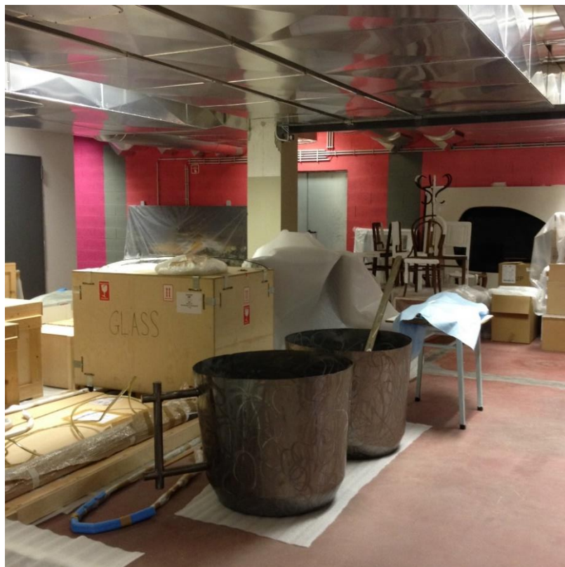
Fig. 32 The view on technical area and the air conditioner power unit of Núcleo de Arte
