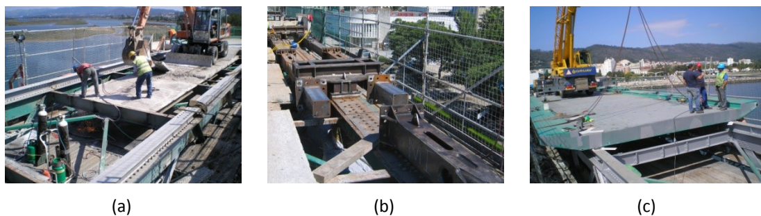
Figure 3.4 – Critical stages of the rehabilitation: (a) top deck removal; (b) strengthening of the top chords; (c) placing a steel module of the road deck.
