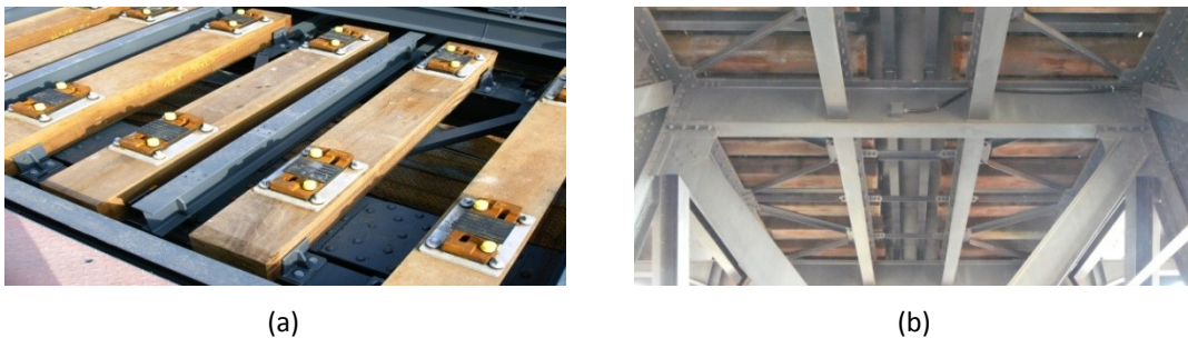
Figure 7.3 – General view of the upper deck of the Luiz I Bridge: (a) top view; and (b) bottom view.
