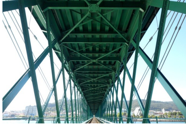
Figure 3.5 – Bottom view of the Eiffel Bridge top deck, after the recent rehabilitation.
