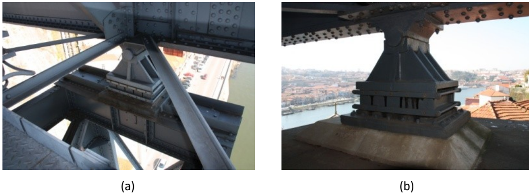
Figure 8.6 – General view of the support bearings installed on the upper deck of the Luiz I Bridge: (a) pillar P3; and (b) pillar P4.
