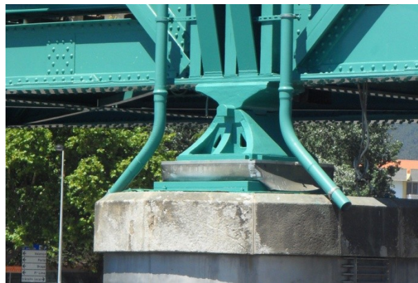
Figure 3.6 – View of a new support bearing.
