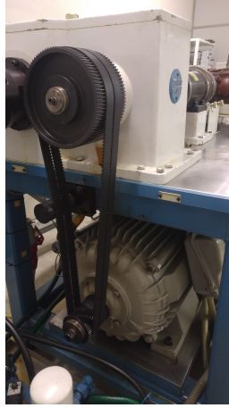
Figure 3.4: 3-phase electric motor and timing belt.
