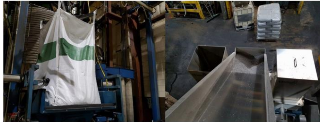
Figure 8 - Bagoff equipment and EPDM tanks
