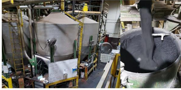
Figure 9 - Silos and mixing process
