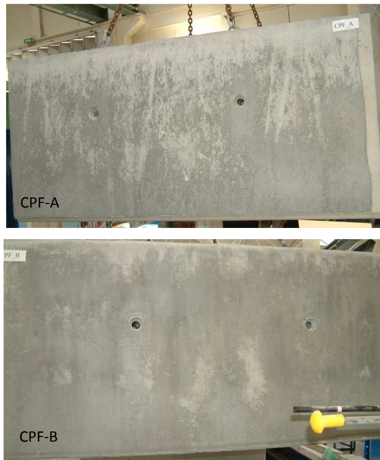
Figure 2.6 – Concrete surfaces resulting from application of CPF-A on CC box-culvert and from application of CPF-B on CC box-culvert.
