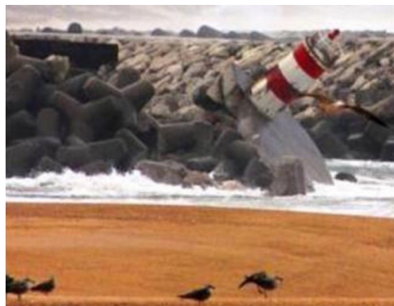
Figure 4.9 - North breakwater head of Nazaré harbour in December 2013, (Ferreira et al. , 2015).
