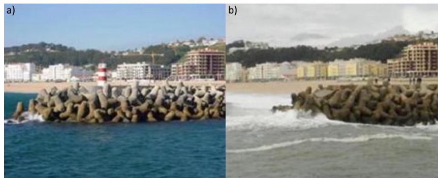
Figure 4.8 - Evolution of the north breakwater's head: a) Before any significant damage; b) Photograph taken on 7 th January 2014, after the two storm events, (Ferreira et al. , 2015).
