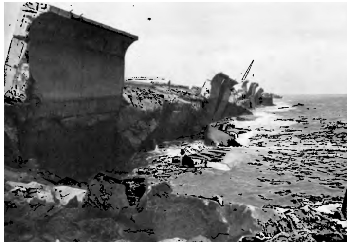
Figure 4.6 - Damage to the crown wall and dolos armour layer, taken immediately after the February 1978 storm, (Baird, et al. , 1980).
