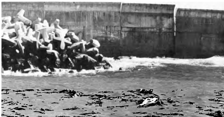
Figure 4.7 - Dolos removed from the front of the seawall, broken dolos and superstructure, (Baird, et al. , 1980).
