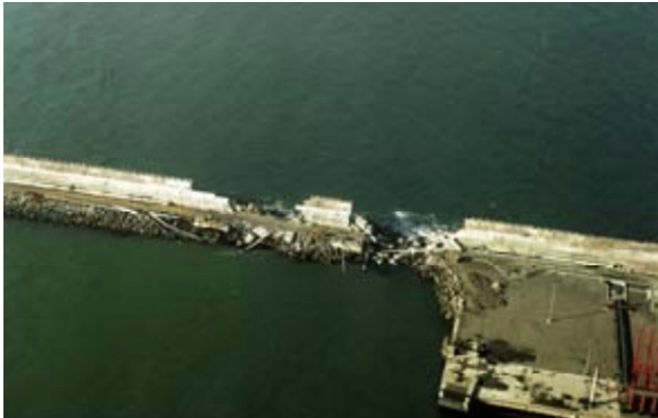
Figure 4.13 - Punta Lucero Breakwater: Port of Bilbao, damage view (Serret et al. , 2010).
