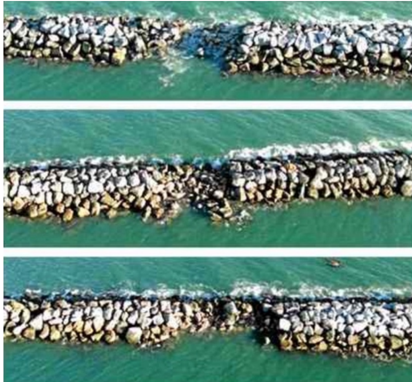
Figure 4.15 - Breakwater of the container Port of Long Beach, United States.
